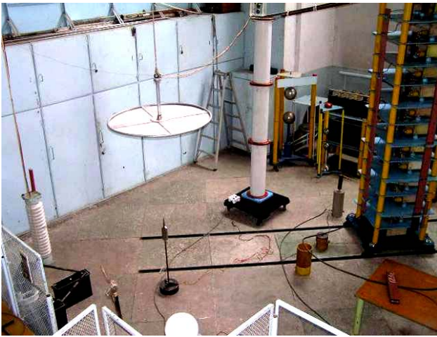
Fig. 9. General view of the high-voltage test stand of the R&DPCI «Molniya» of the NTU «KhPI», intended for testing lightning protection equipment of technical objects with commutation aperiodic voltage pulse with amplitude up to \pm 1 MV of time shape 250 \mu\text{s}/5000 \mu\text{s} and containing in the scheme a mobile superhigh voltage capacitor voltage divider of the type CDV-1, 2 [16]
