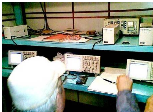
Fig. 5. External view of the placement of three Tektronix TDS 1012 digital storage oscilloscopes that register in parallel useful electrical signals from one SC-300M1 measuring shunt in a buried screened measuring hopper designed for metrology support of field testing of various technical objects for lightning resistibility [9]
