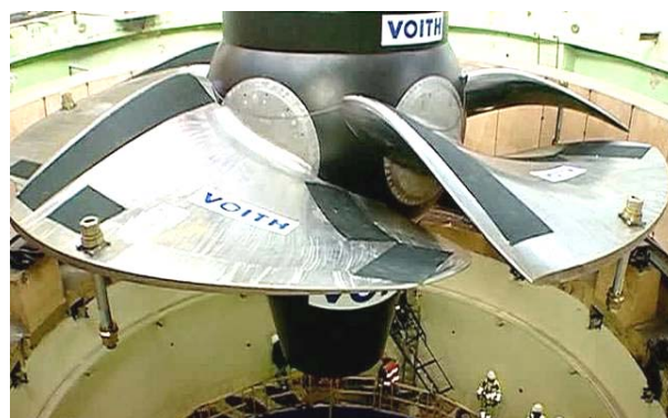
Fig. 4. General view of the new modern powerful rotary-blade hydraulic turbine at the time of its installation at the HPP [7]
