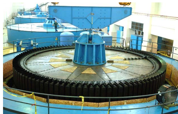
Fig. 8. General view of the machine hall of a powerful HPP at the moment of lifting the rotor of one of its large-sized hydraulic electric generators of vertical design [4]
