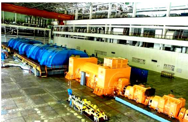
Fig. 12. General view of the power plant hall of the power unit with the thermal power of 1000 MW of the South-Ukrainian NPP [17]
