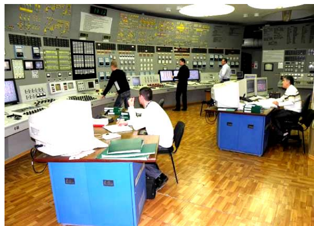
Fig. 13. General view of the block control panel (separate specific «command post») of one of the power units with thermal power of 1000 MW at the South-Ukrainian NPP [17]
