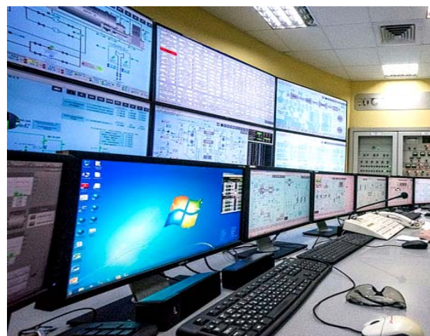
Fig. 7. General view of the control panel of a modern high-power TPP [15]
