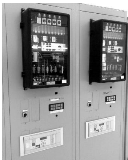
Fig. 24. Distance protection of lines based on MPD type MiCOM P437 (bottom) and on electromechanical type LZ-31 (top) connected in-parallel
