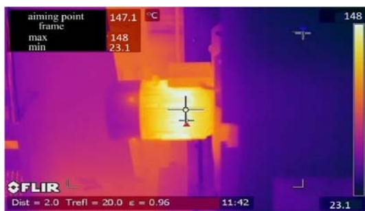
Fig. 3. A thermogram of the induction generator
