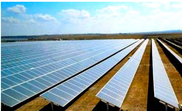
Fig. 16. General view of a fragment of the territory of the SPP «Perovo» with installed power of 100 MW (Crimea) [18]
