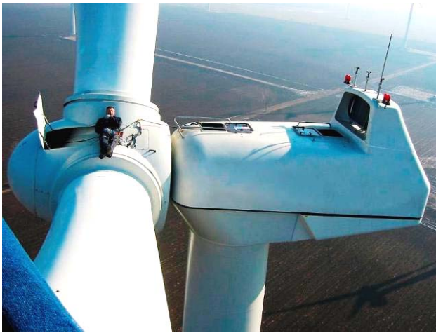
Fig. 5. A rare photo of the moment of service at altitude of about 70 meters and the turbine rotor blades of modern land-based horizontal-axis three-bladed wind turbine installed capacity of up to 1500 kW [11]
