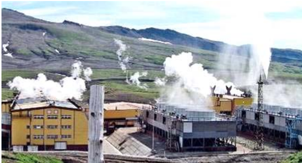
Fig. 22. External view of Mutnovskaya GTPP with installed power of 50 MW (2002, Kamchatka, RF) [22]
