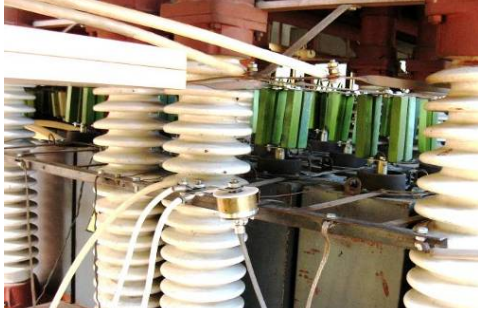
Fig. 13. General view of a high-voltage measuring shunt of the ShK-300M1 type, connected to the collector of a high-current discharge circuit of a powerful UITOM-1 type PSG
