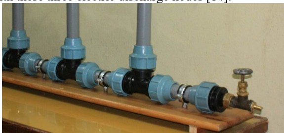
Fig. 4. A photograph of a tubular system with these three electric discharge nodes
