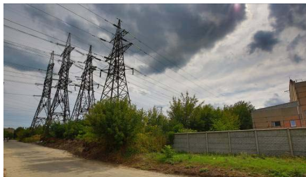
Fig. 1. Group of high voltage power lines
