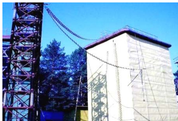
Fig. 11. General view of GSVP of GKIN-2 type, which forms a standard aperiodic switching pulse of voltage of a temporary shape T_g/\tau_p \approx 205/1900 \mu\text{s} with amplitude U_m up to 2 \text{ MV} on the tested electric power facility (the modernized generator GIN-4 is placed on the right, and an insulating support 11 m high with load capacitance C \approx 13.3 \text{ nF} for 3 \text{ MV} , to the upper potential electrode of which from the GIN-4 generator forming R_f \approx 4.28 \text{ k}\Omega and from the load capacitance – current-limiting R_l \approx 4.59 \text{ k}\Omega resistors are connected) [24]
