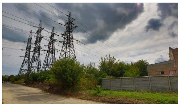
Fig. 1. Group of high voltage power lines
