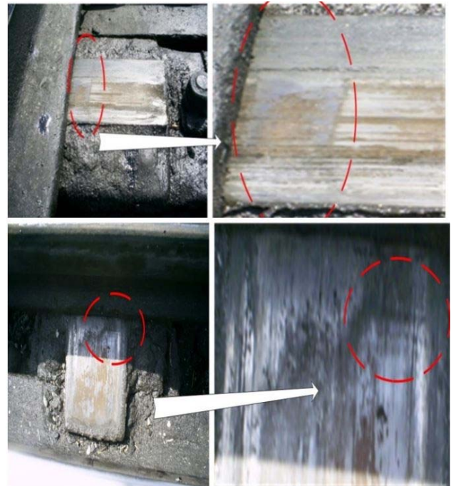
Fig. 10. State of the switching surfaces
