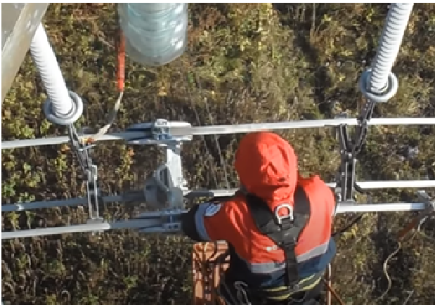
Fig. 1. Execution of repair works by NPC «Ukrenergo» on the 330 kV power line under voltage
