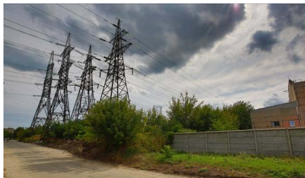
Fig. 1. Group of high voltage power lines
