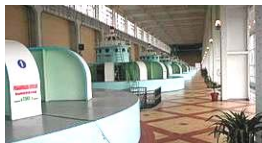
Fig. 11. Modern view of the hydraulic turbine hall of the Dneprovskaya HPP with installed power of 1548 MW [15]
