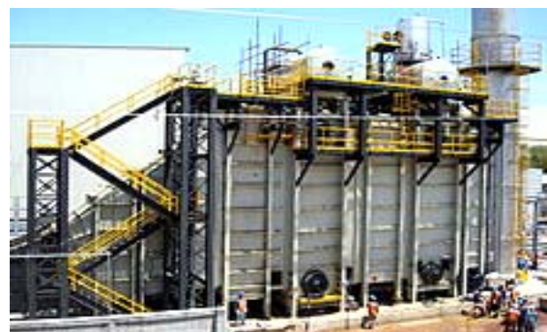
Fig. 2. General view of heat recovery boiler of the GTPP [7]
