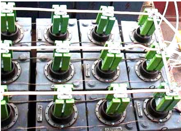
Fig. 25. General view of a fragment of a powerful high-voltage CES single module performance at a rated voltage of \pm 50 kV and rated stores electric energy 420 kJ with its parallel-connected capacitors type ИК-50-3 in the amount of 112 pieces. and rigidly mounted on their findings of high-volume constant high voltage protective graphite-ceramic resistors TBO type-60-24 \Omega [49]
