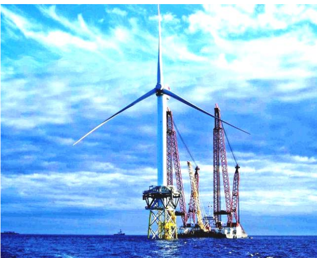
Fig. 7. Moment of preparation for assembly work on the modern sea-based three-bladed horizontal axis wind turbine installed capacity of up to 600 kW [11]
